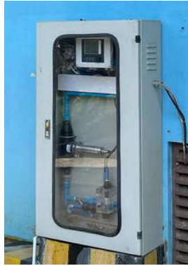
Gambar 4. 4 Residual Chlorine Automatic (RCA)
