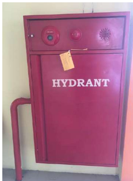
Gambar 4.8 Fire Hose Box
