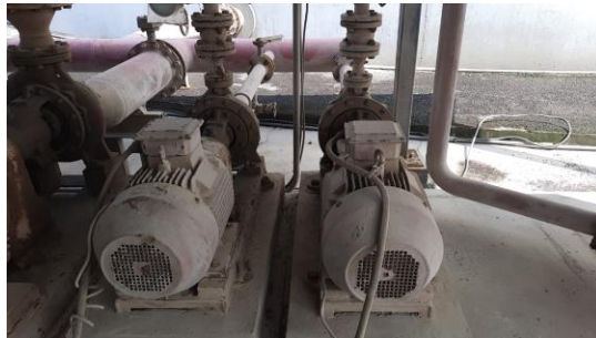
Gambar 4.10 Pompa Jockey Hydrant
