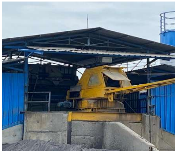
Gambar 1. Area Batching Plant Jalur II
