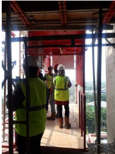
Inspeksi Passenger Hoist
