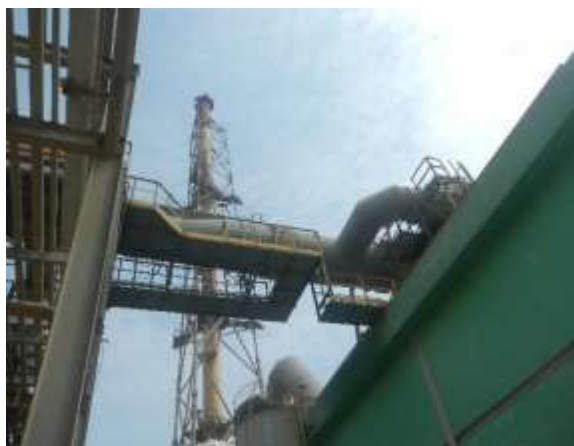
Cerobong asap / stack
