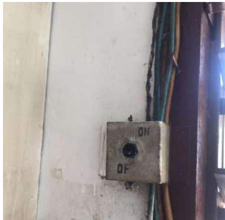
4.9 Gambar alarm sirine manual
