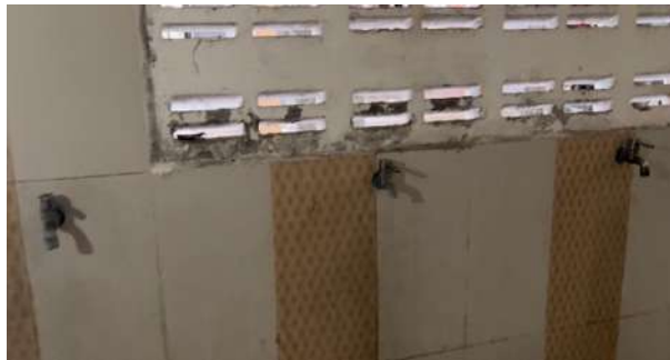
Gambar 4.29 Kran air wudhu Masjid Riyadhus Salma
