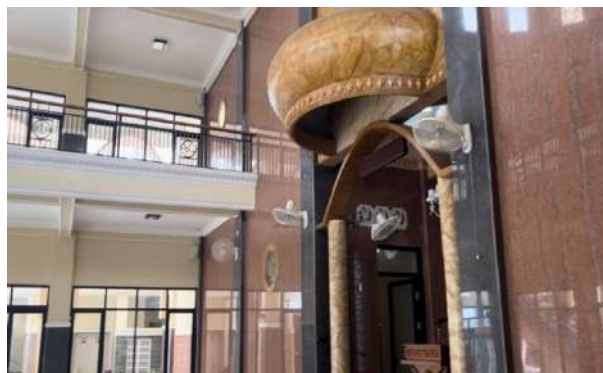
Gambar 4.16 Kondisi dinding Masjid Riyadhus Salma
