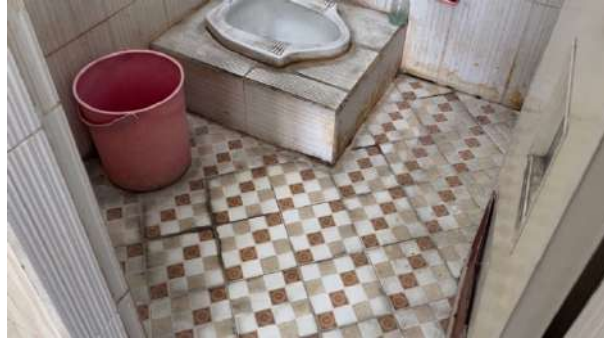
Gambar 4.34 Kondisi toilet/WC Masjid Riyadhus Salma
