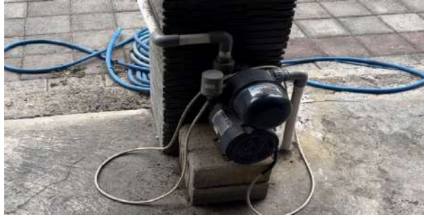
Gambar 4.28 Pompa air Masjid Riyadhus Salma
