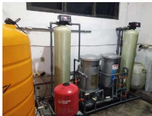
Gambar 4.2 Water Treatment di Lokasi 1
