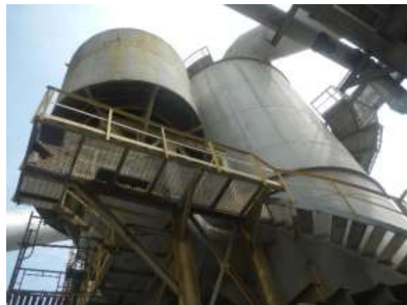
Gas Scrubber di pabrik III Asam Sulfat
