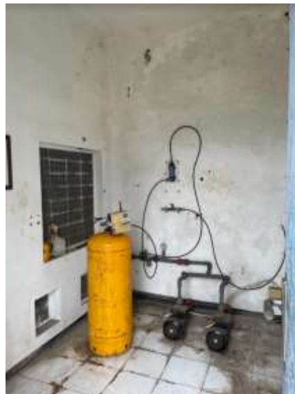
Gambar 4. 11 Ruang Chlorinasi Reservoir Bangkon
