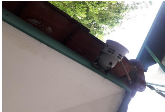
Gambar 4.3 Emergency Alarm Sumber: Hasil Observasi, 2019
