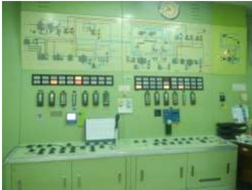
Gambar 1. Control Room Effluent Treatment
