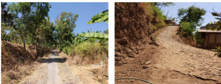
Figure 1. Road condition of Sawahan district
